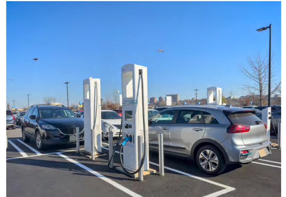
Figure 15. Electric Vehicle Charging
